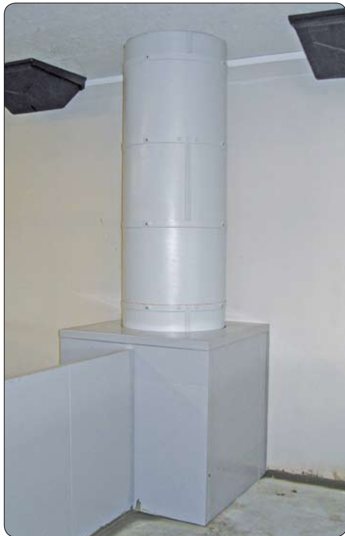
The old equipment box, which was located completely up against the wall.
