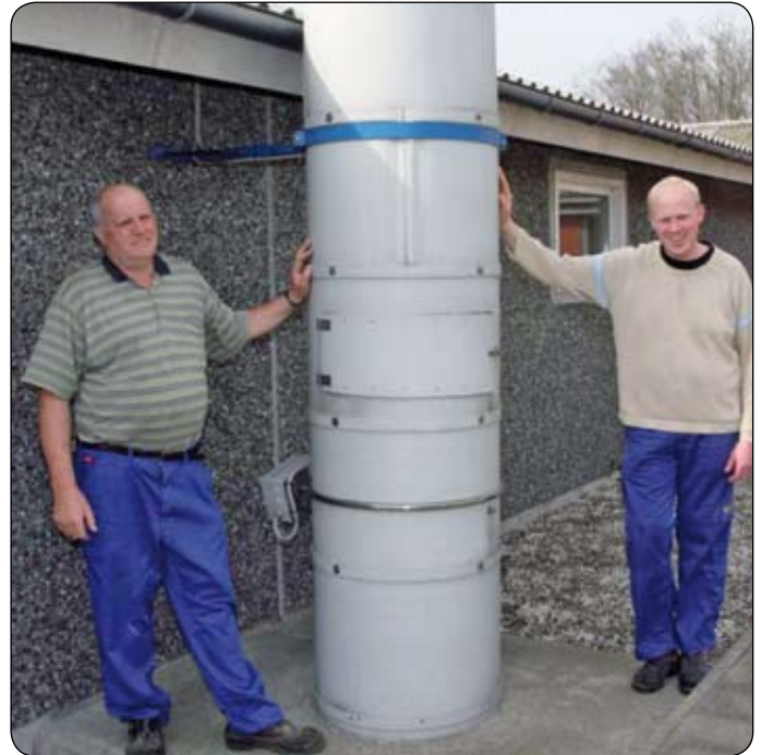
Poul and Ole Jensen have underfloor exhaustion in most of their houses and there is no doubt in their minds that they prefer being in houses with underfloor exhaustion. Photo: Pressebureauet Århus.
