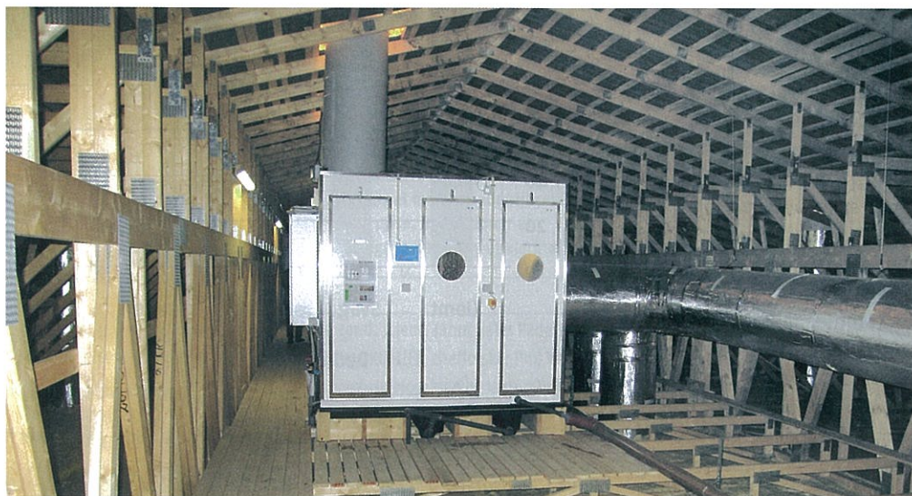
Luftrenseren Farm AirClean BIO System fra SKOV A/S.
